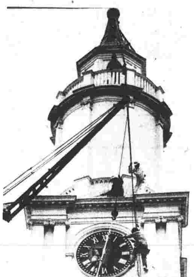
Workers install seven-foot faces at Old First Church in Court Square in Springfield, Mass., Tuesday. Built in 1819, the church is the oldest wooden public building in Springfield, and has had no clock since 1900. (UPI photo)
